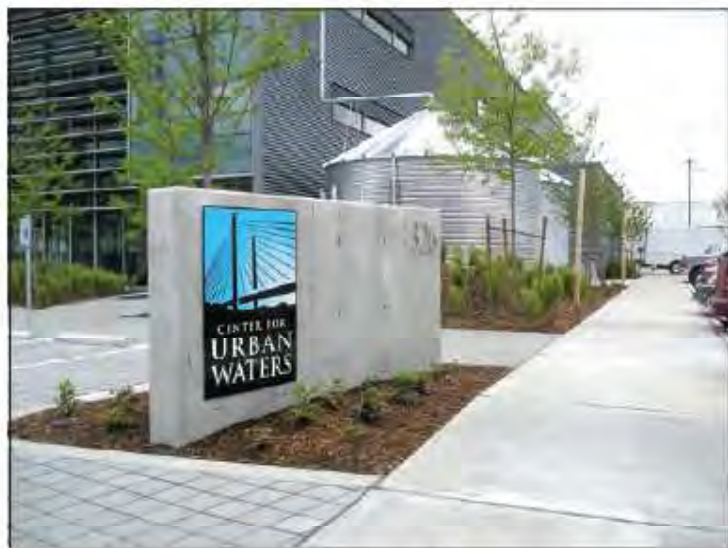
Eagle Harbor Mechanical installed a rainwater harvesting system in Tacoma, WA's Center for Urban Waters building, relying on Jay R. Smith Mfg. Co.® products to do the job. The visible stainless steel water storage tanks draw attention to rainwater harvesting and the city's efforts to promote sustainability.
