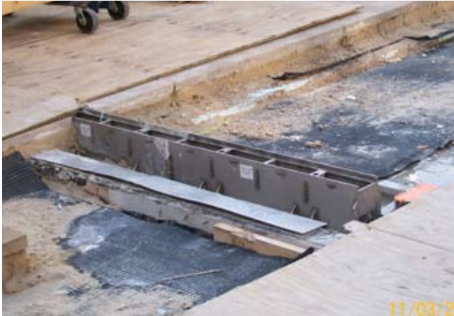
Pre-assembled, fabricated Trench Drains by Jay R. Smith Mfg. Co. installed at The Lincoln Center.
